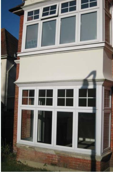
UPVC Replacement windows mar this fine façade
