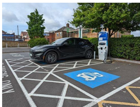
Photo: Recently installed charging point at Westhill car park
